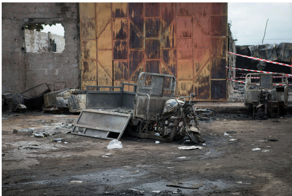
The burned-out remains of an informal fuel warehouse in Sèmè-Kraké, following a fire that claimed 35 lives, September 2023.
